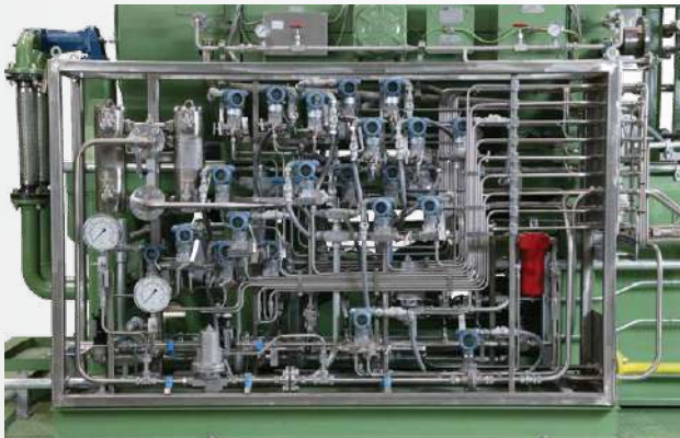
Gas seal transmitter rack with 2-of-3 voting, seal gas filtering and purge gas filtering
