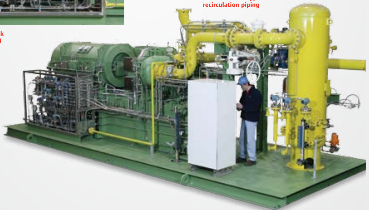
Fuel gas booster skid with scrubber, bypass and recirculation piping
